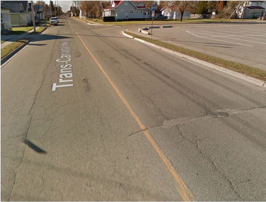
Poor: Pavement is in poor condition with frequent patterns of moderate defects. Rideability is poor, and surface is rough and uneven.
