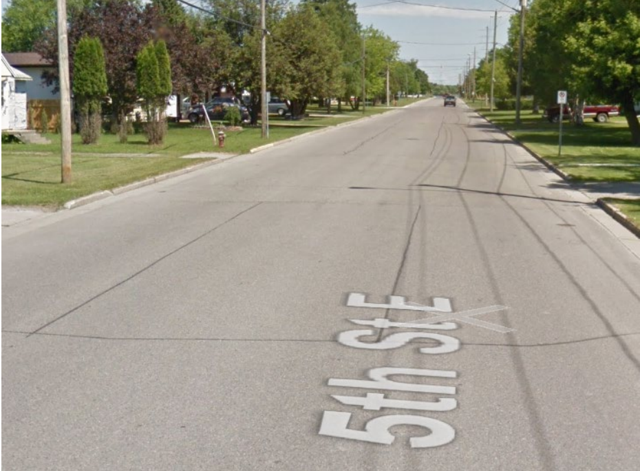
Fair: Pavement is in fair condition with intermittent patterns of slight to moderate defects. Rideability is fair, and surface is slightly rough and uneven.
